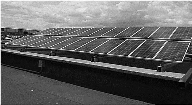
Figure 4. Installed solar panels Source: Taken from fieldwork.
